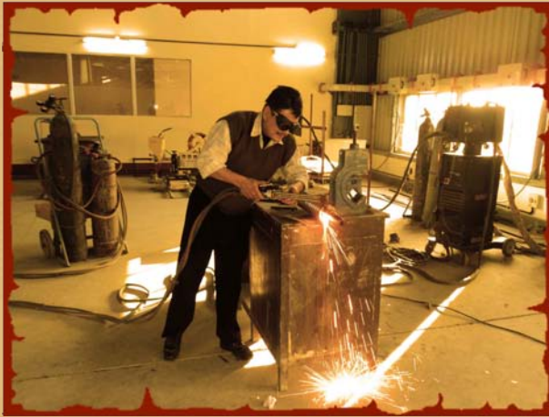
Gas cutting by oxidizing flame which contains acetylene gas and excess of oxygen
